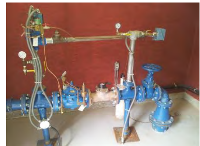
Well 3, backup, 50 hp with genset
