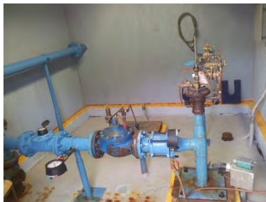
Well 2, lead, 30 hp
